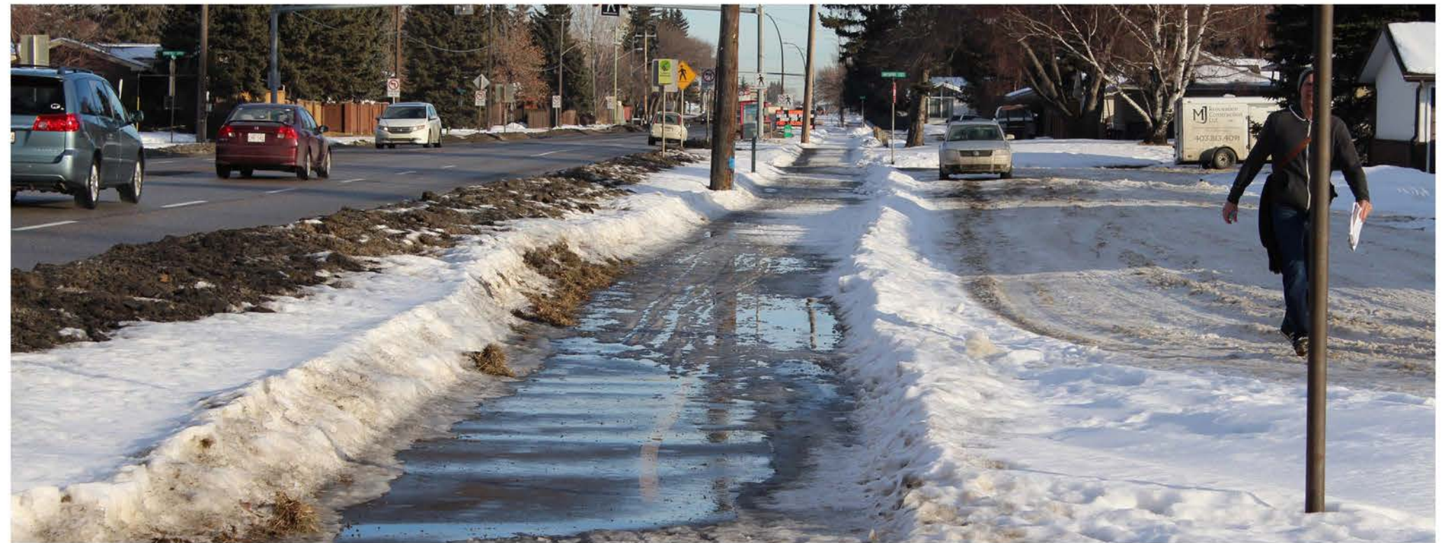
Existing conditions of Heritage Drive pedestrian infrastructure. Note poor drainage forcing pedestrians to walk on adjacent residential road.
